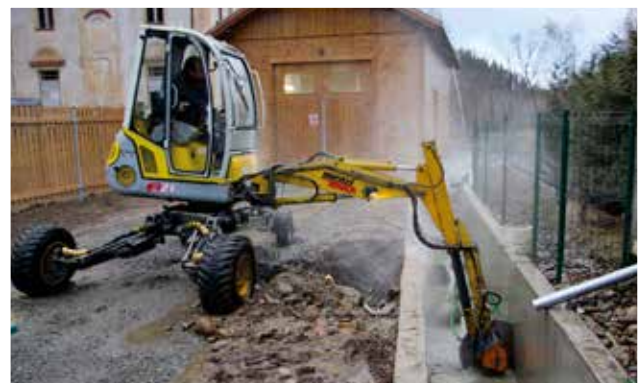
📍 Echidna D1 diamond rocksaw cutting expansion slot in reinforced concrete water channel. (Stachy, Czech Republic)
